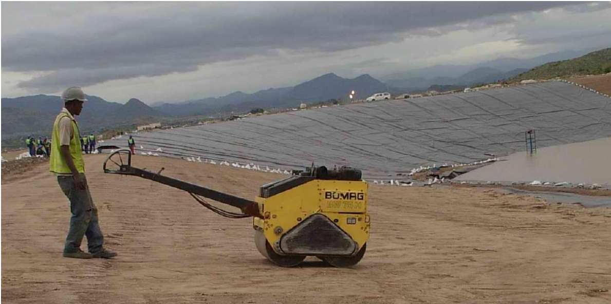
Figure 5: Construction taking place on the TDF showing the compacted soil layer beneath 1.5mm HDPE liner
