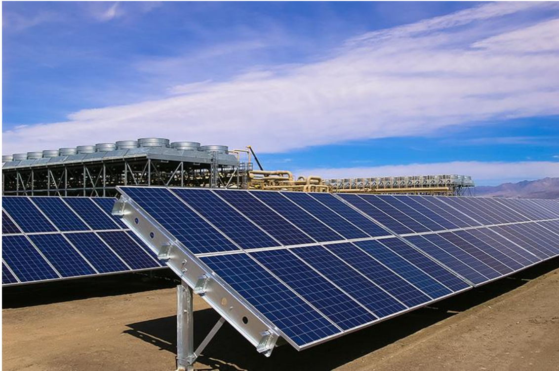
Figure 1.3: Photograph of PV facility (Borthakur, 2017).
