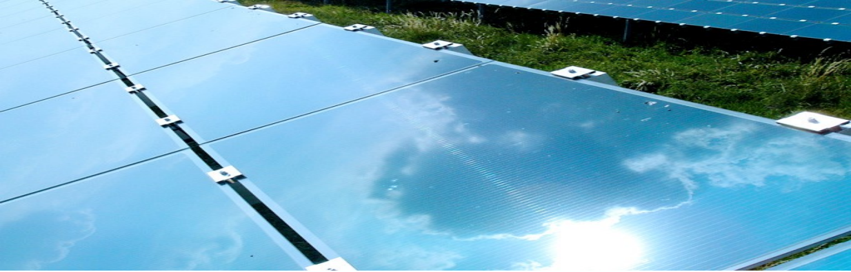
Figure 5. Close up of a Solar Photovoltaic Panel
