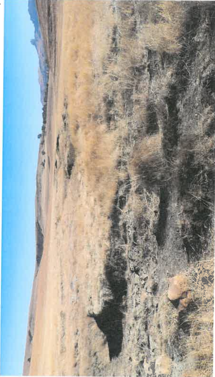
Figure 13: Example of a stream crossing (severe erosion) with poorly constructed road – needs rehabilitation.
