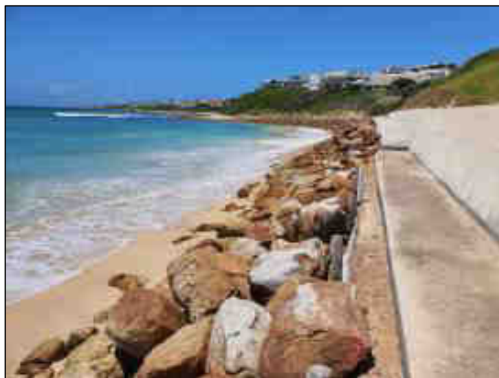
Figure 3-8: View farther rock revetments and concrete reinforcements along the St Francis beach frontage.
