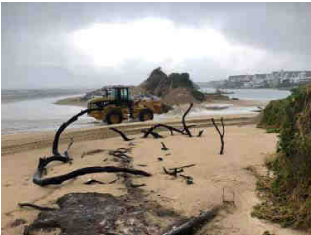
Plate 6.5 Front end loaders reworking the beach material to repair the breach in the spit (SFPO NPC)
