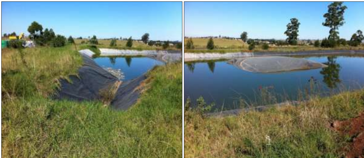
Figure 2.1 Existing oxidation ponds at St Patrick's Hospital. Left: inlet; Right: an air bubble developed indicating leakage in the lining of the pond.
