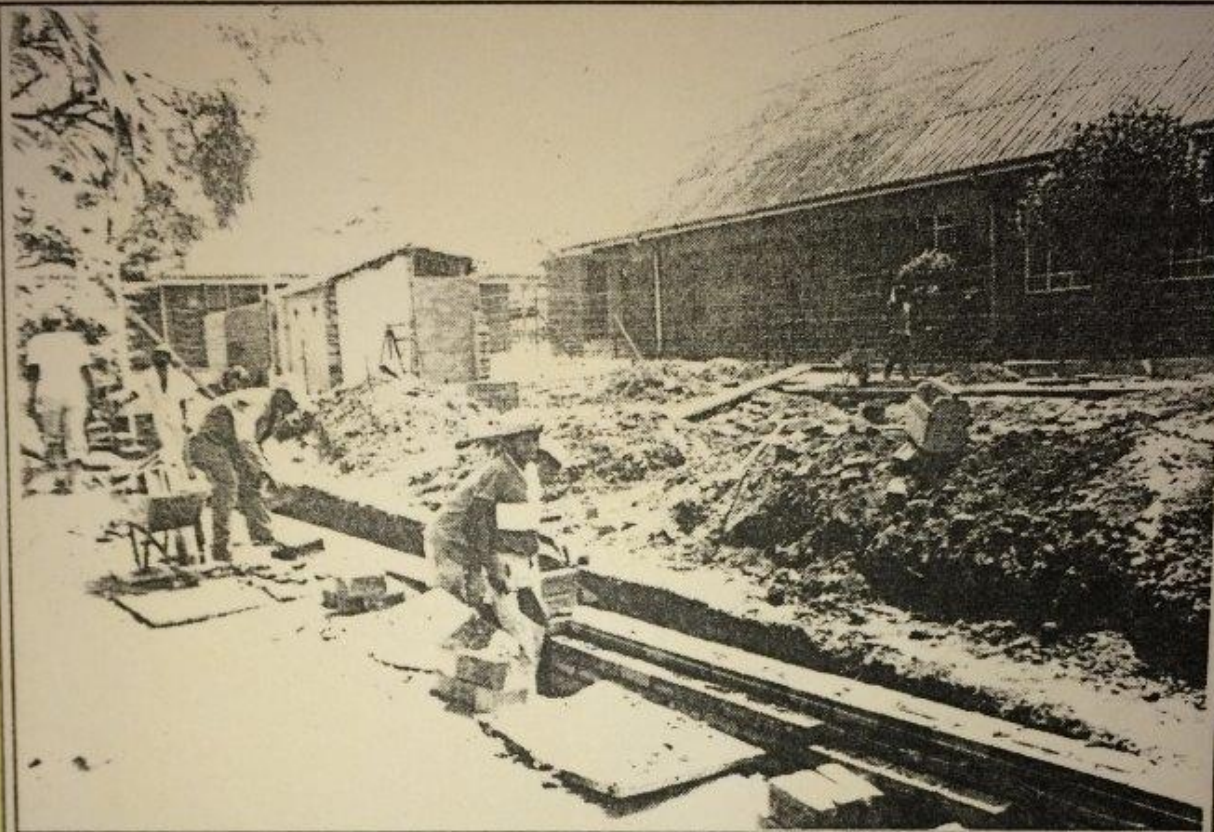
Construction workers busy on site at the Stanger Secondary School which is on schedule.
