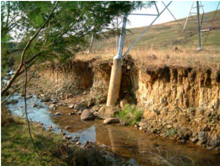
Figure 8. Example of the dangers of erosion to power lines (photo Jorge Correia)
