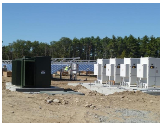
Figure 5: Inverter (Photo courtesy of BlueWave Capital SA)
