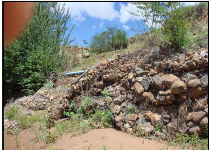
Figure 15: Gabions collapsed at river bank
