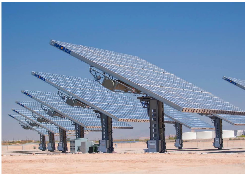
Figure 2.10: The support structures elevate the panels by 15 m and allow for dual axis tracking of the sun for increased efficiency (Source of Amonix™)
