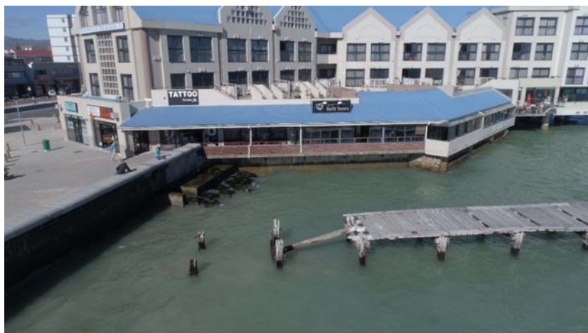
Figure 1: The Jetty after the shoreward section was removed, and the revetment constructed (2021).
