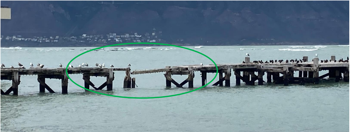
Figure 6: Loose and partly detached support beams to be removed (Section D). Remaining decking needs to be inspected up-close and any rotten/partly or fully detached planks to be removed.
