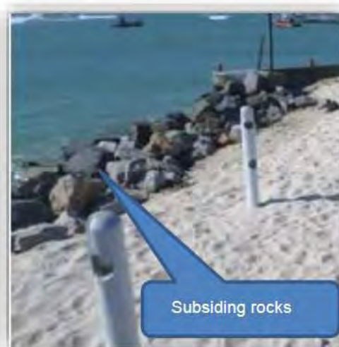
Figure 11: Subsiding of rock revetment
