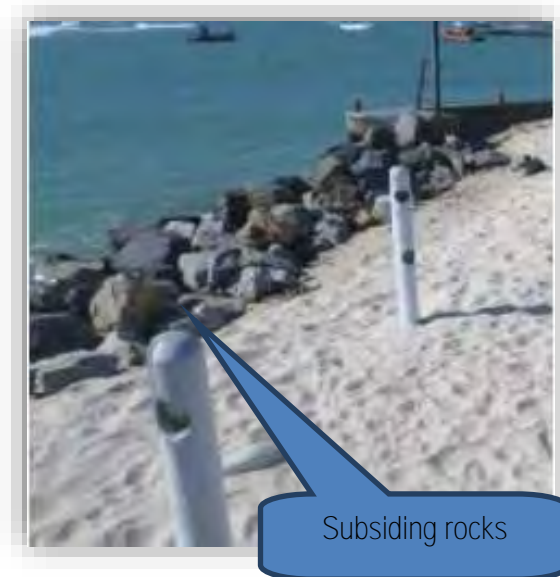
Figure 9: Subsiding of rock revetment
