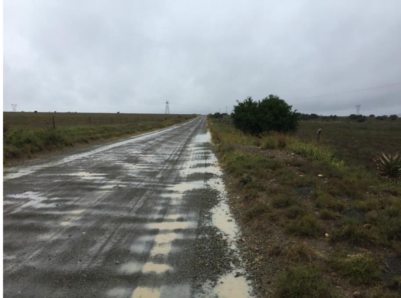
Figure 3 – Condition of District Road DR02054
