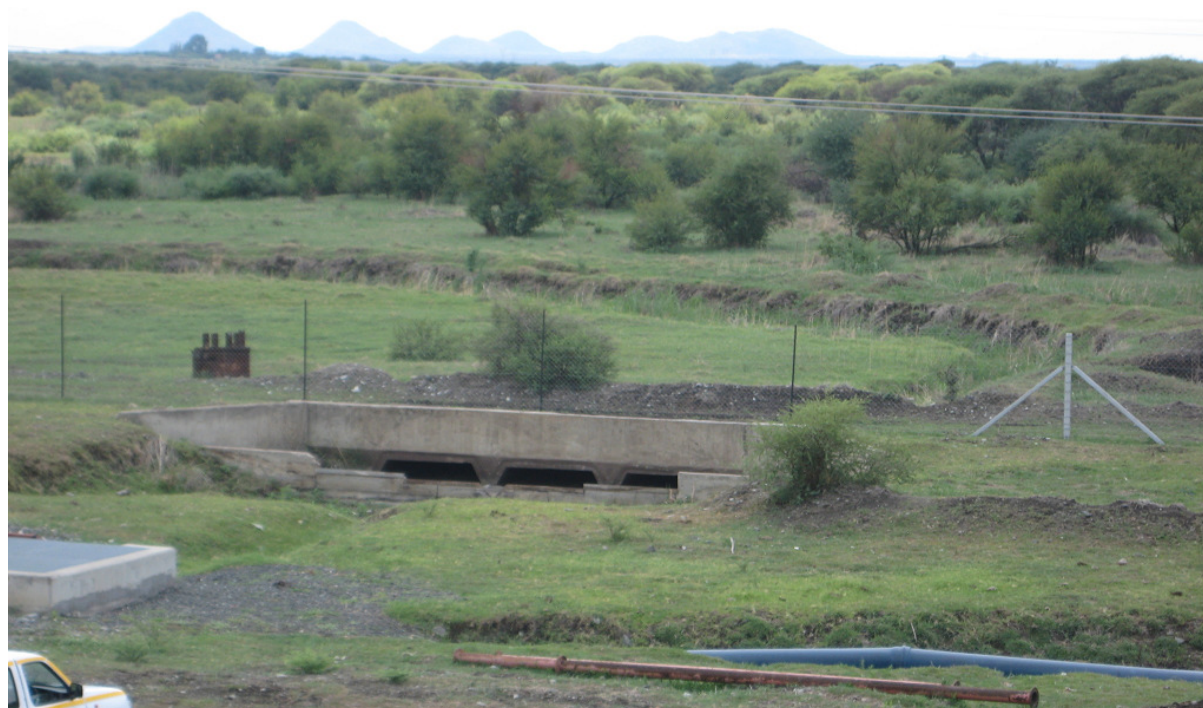
FIGURE 2-3: UNION MINE DISCHARGE POINT (25 FEBRUARY 2016)
