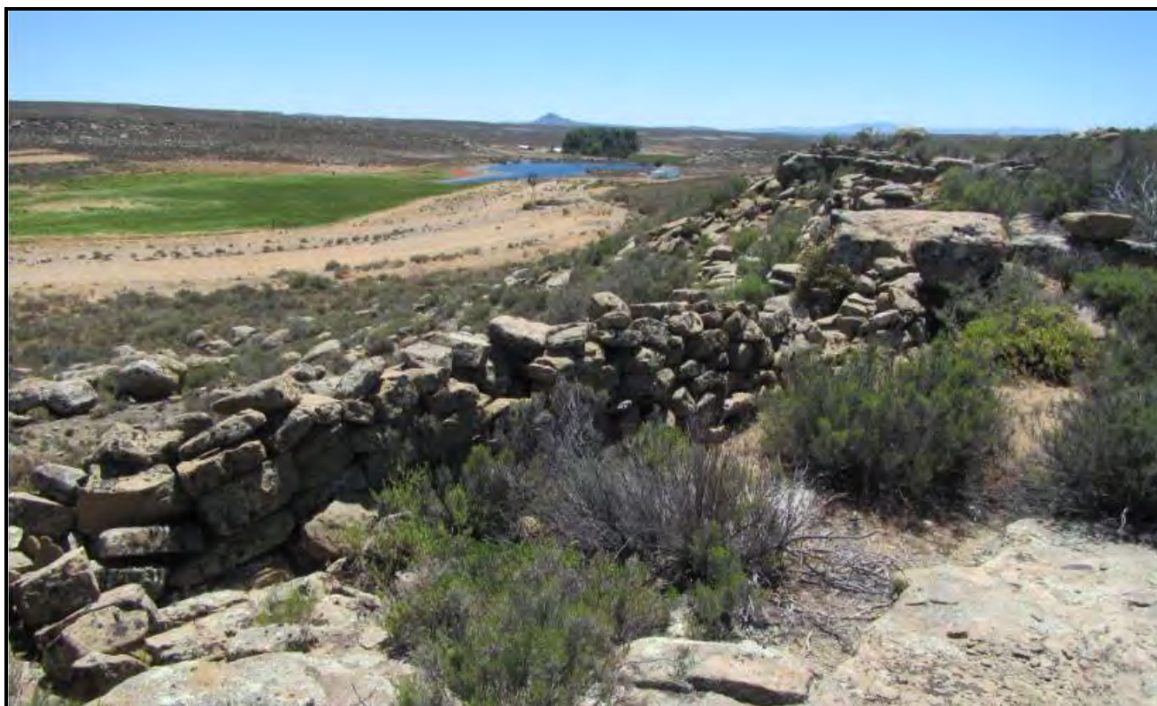
Figure 35: View towards the northeast showing the wall and part of its enclosed lands.
