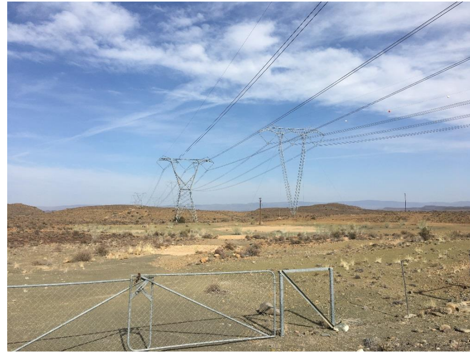
View of the existing Eskom power lines south of the proposed 400 kV power line, just outside Merweville in the Western Cape (Source: Shawn Johnston).
