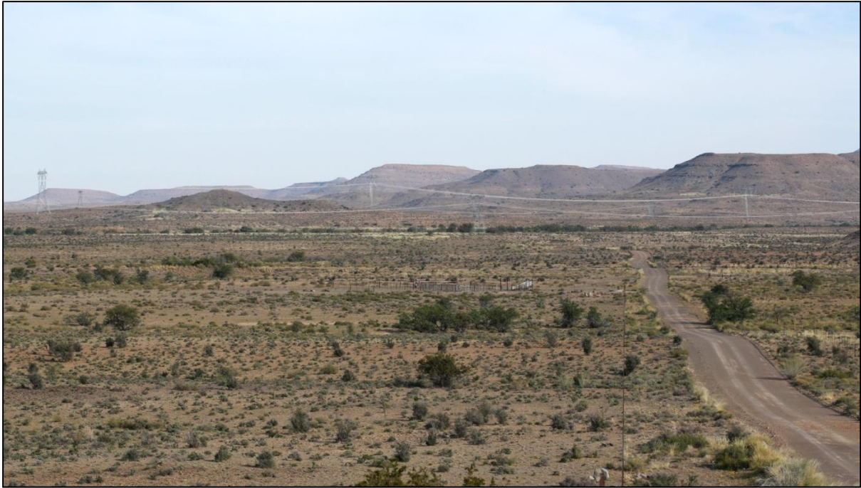
Figure 6. Looking south along the final section of the 132kV line, with the Eskom 400kV lines in the distance.
