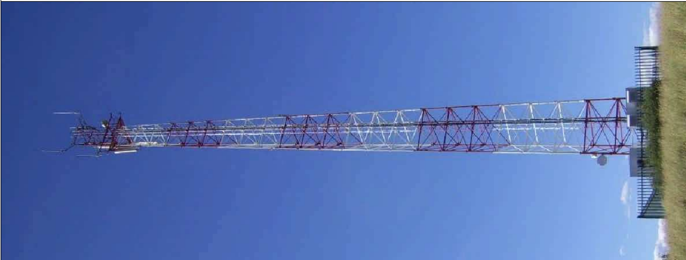
TYPICAL 3-LEGGED LATTICE MAST (PAINTED RED AND WHITE)
