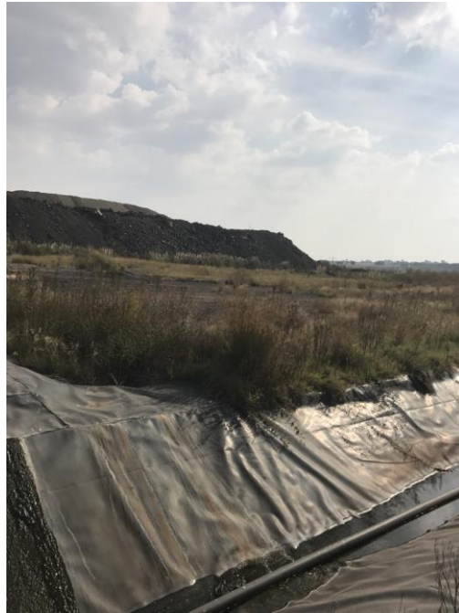
Leachate and storm water channeling towards collection facility
