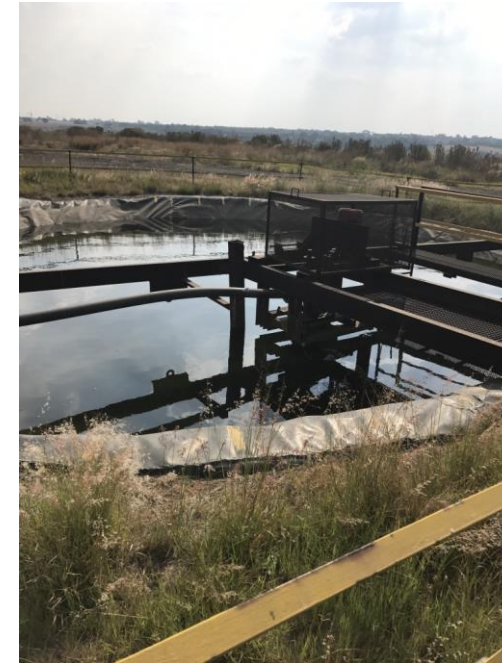
Leachate and storm water collection facility (RWD)
