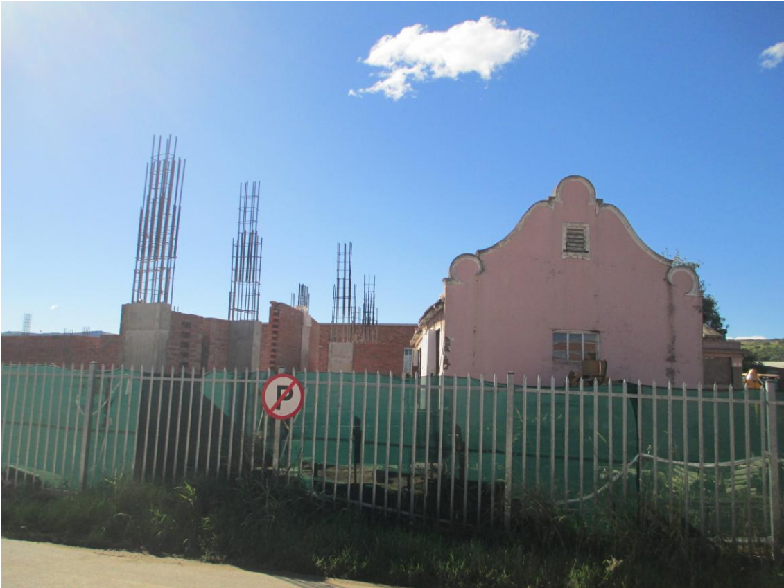
SOUTH AND PARTIAL VIEW OF THE WEST FACADE AND THE NEW BUILDING: THE OPENING ON THE WEST FACADE WHICH USED TO LEAD INTO THE ADDITION THAT WAS DEMOLISHED WERE OF CONCERN TO AMAFA AND WERE NOT EXPLAINED IN THE INITIAL APPLICATION.
