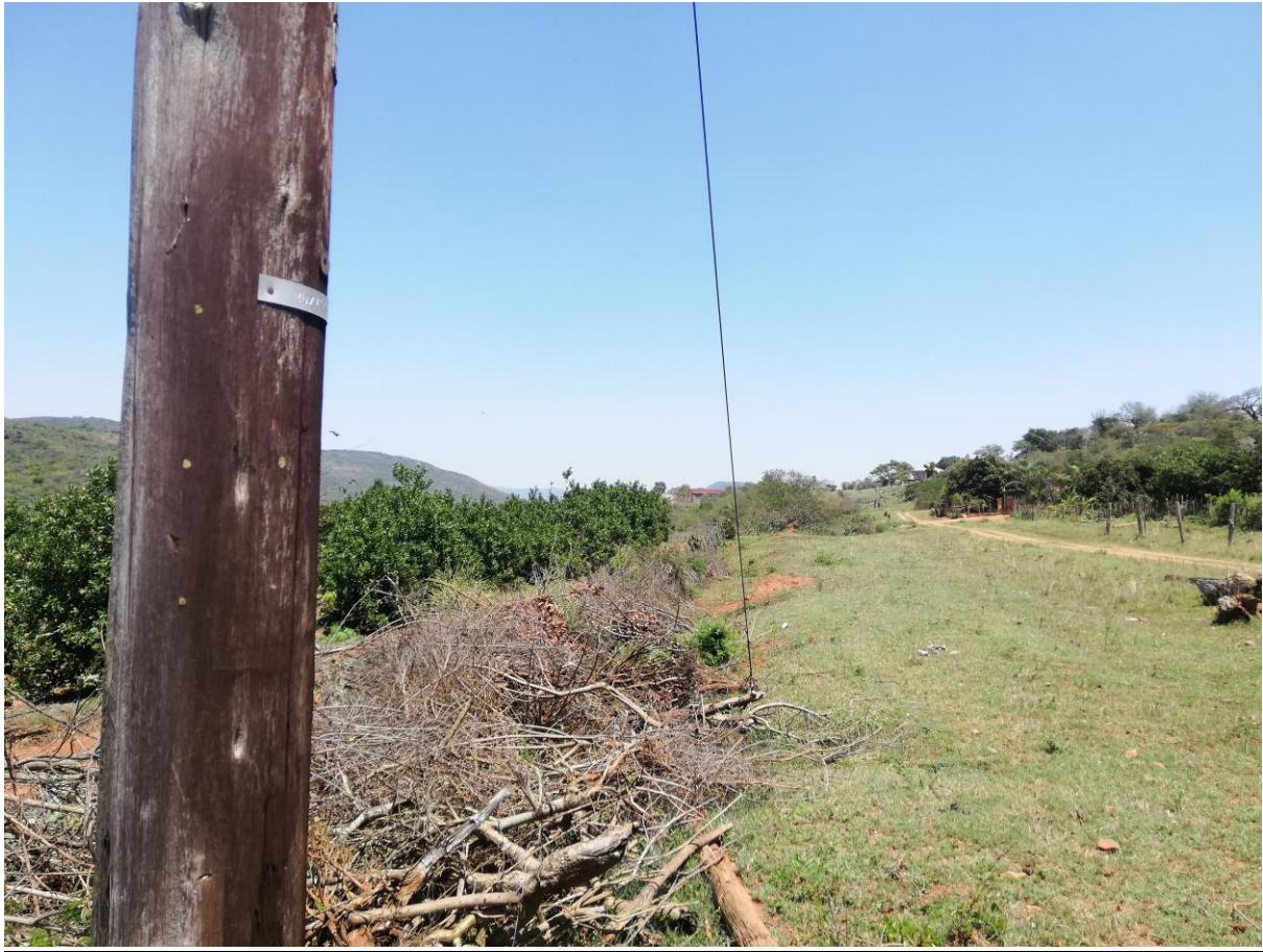
Figure 2 The T-off Pole. The line runs to the left of the small dirt road shown in the picture.
