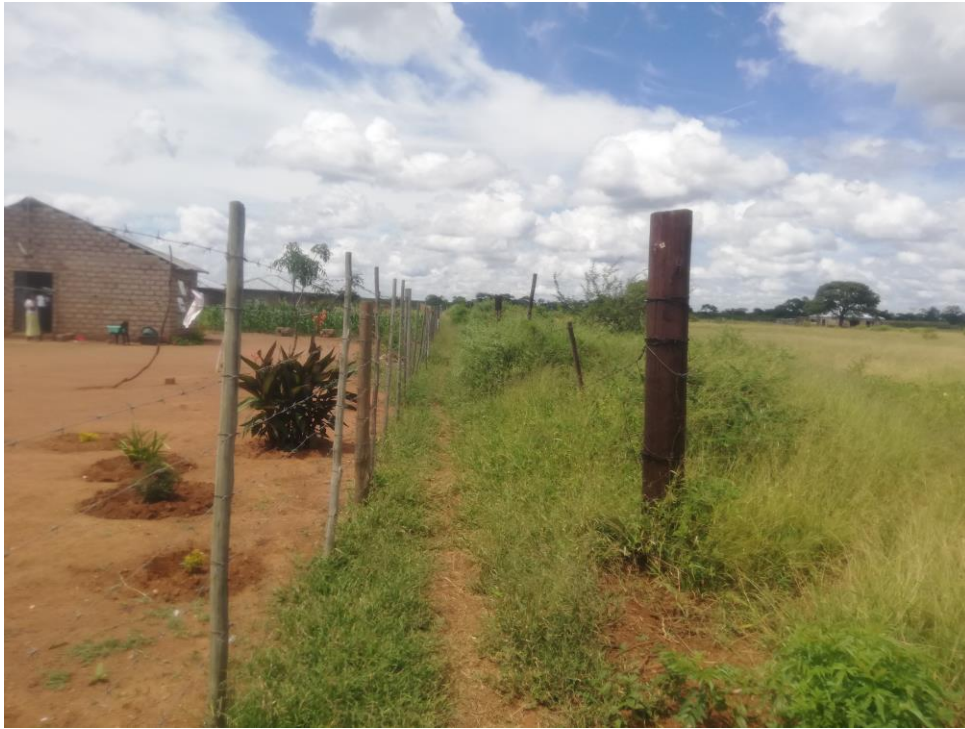
Figure 7 The line runs between the two fences and connects in the customer's yard.
