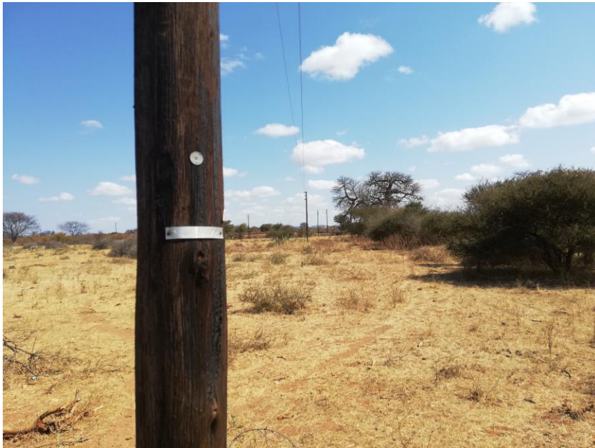
Figure 1 Existing power line
