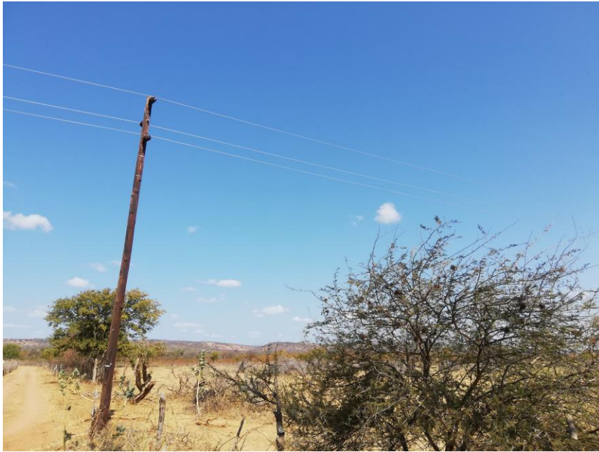
Figure 3 The T-Off Pole. The line runs to the right of the gravel road shown in the picture above
