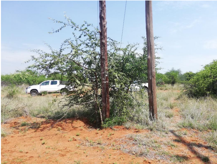
Figure 1 T-off point – The line runs on the left of the structure shown above
