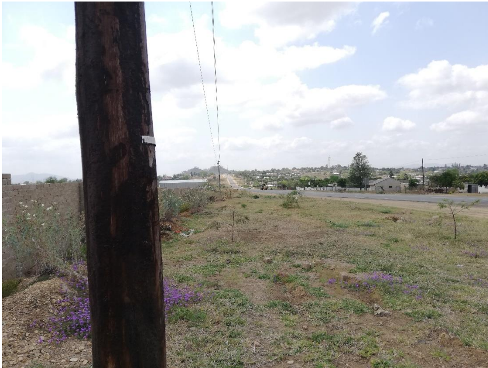
Figure 1 The T-Off point HMJ93A from an existing power line and a provincial road
