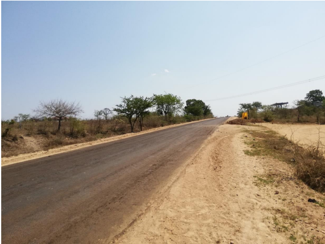
Figure 3 The power line runs to left of the tar road which is under construction
