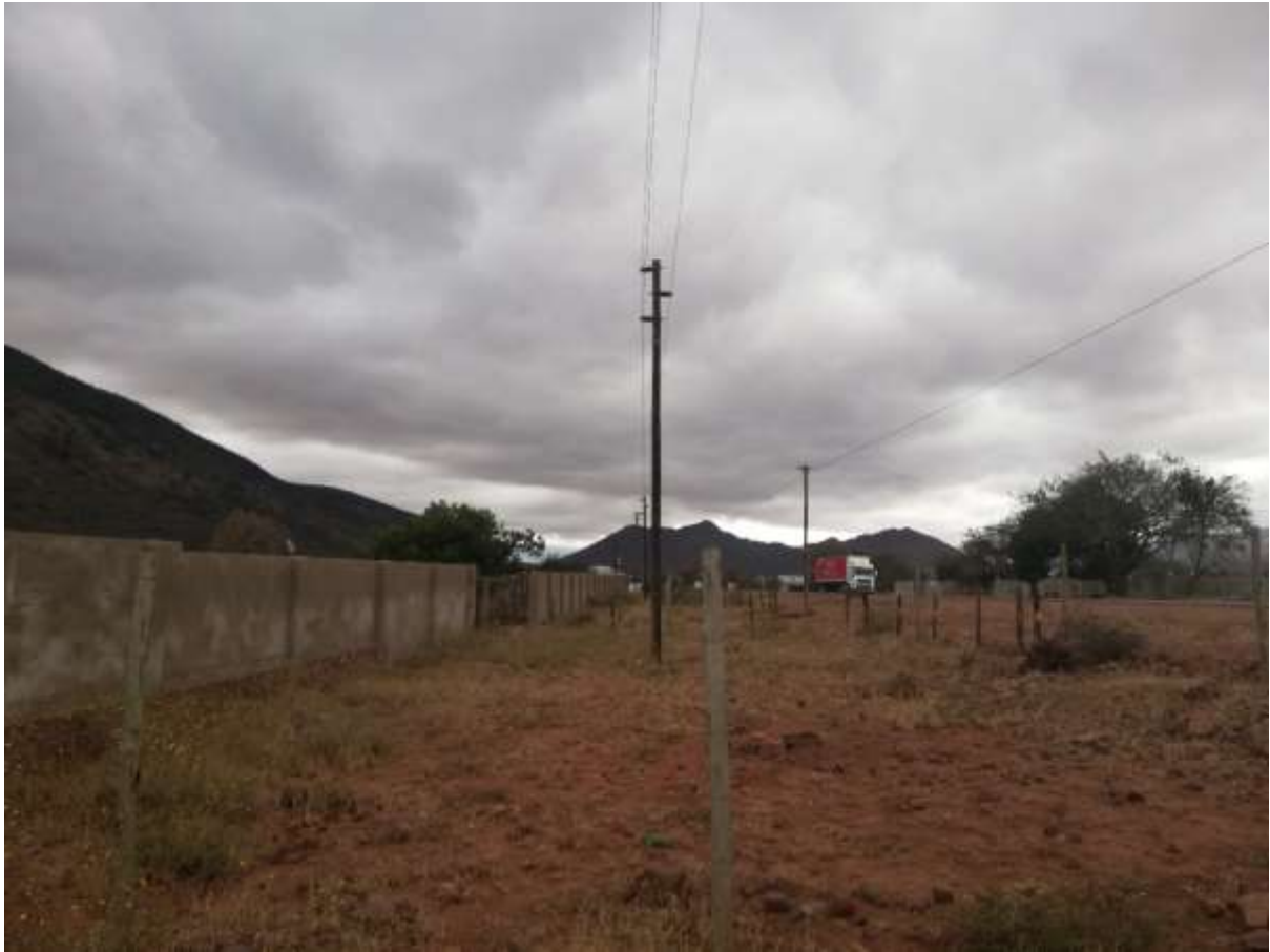
Figure 8 The line connects to an existing medium voltage power line.
