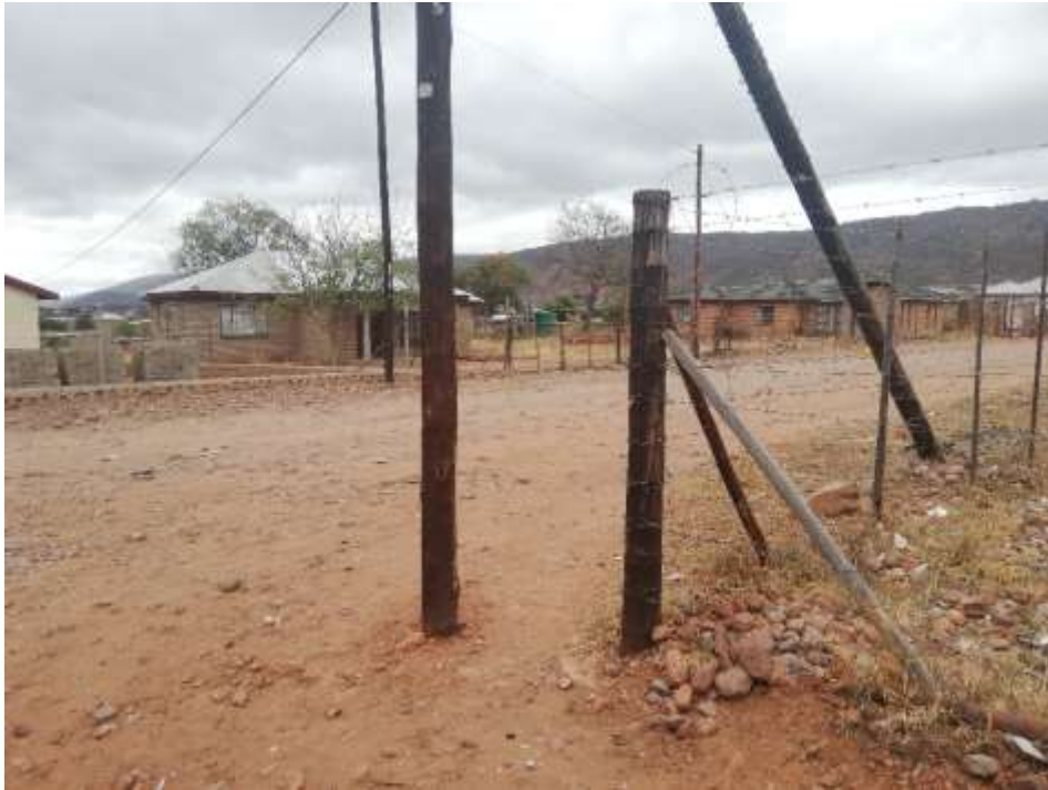
Figure 5 Pole position along the LV power line
