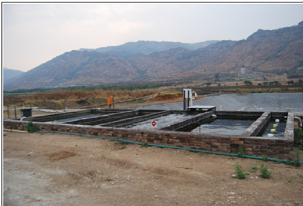
Photo 3.7 Sewage Plant at the Concentrator Plant
