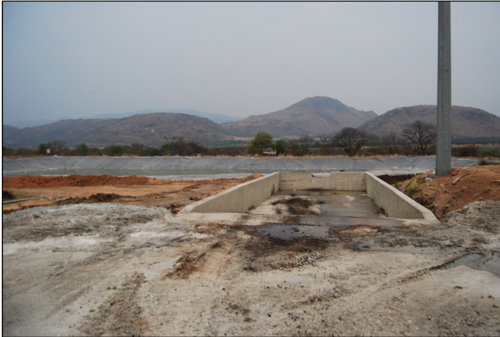
Photo 3.3 New PCD at the North Decline, prior to Operation
