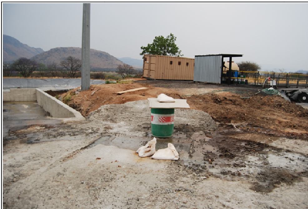
Photo 3.6 Sewage Package Plant at the North Decline
