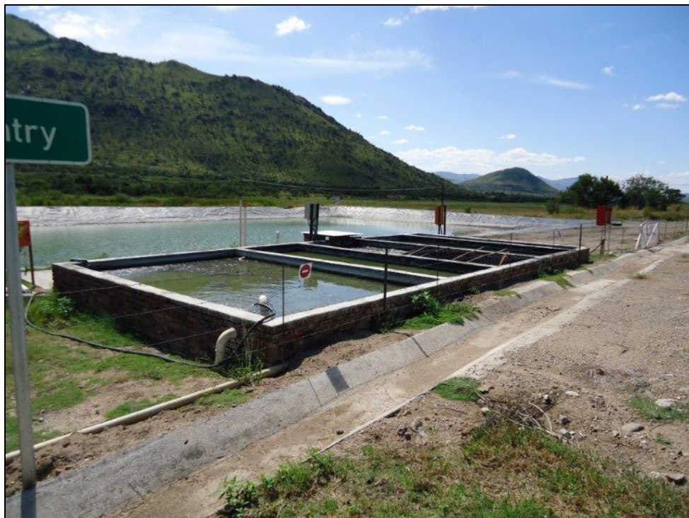
Photo 3.3 Existing wastewater (sewage) treatment plant at the TRP Plant
