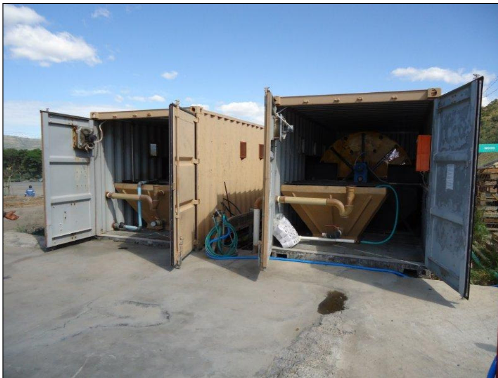
Photo 3.1 Existing wastewater (sewage) treatment plant at the TRP North Decline
