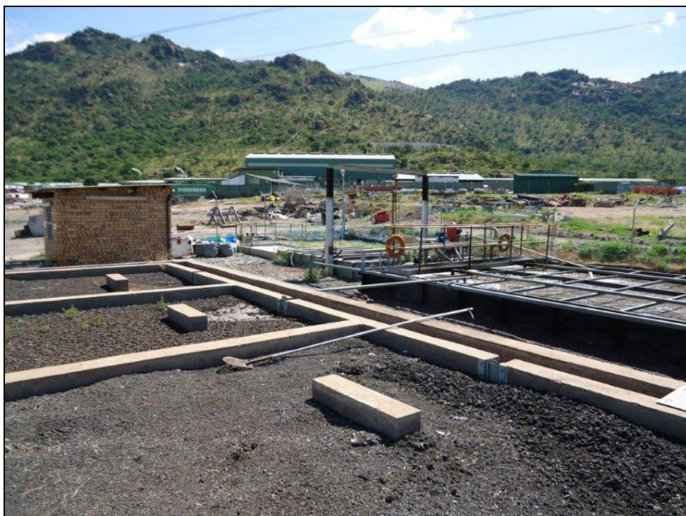
Photo 3.2 Existing wastewater (sewage) treatment plant at the TRP Main Decline
