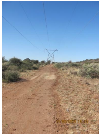
Figure 11: 132kV wooden-lattice power line from west, forming the southern boundary of the proposed solar site.
