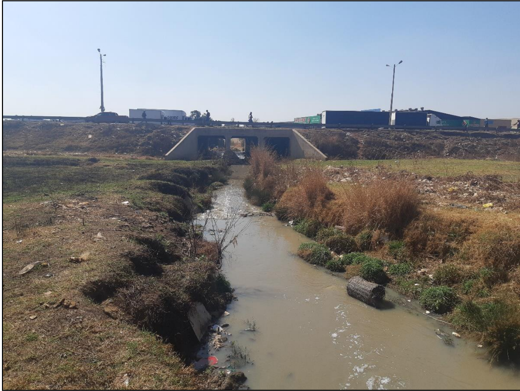
Figure 3: A tributary of the Kaalspruit River flowing beneath the R562 (Olifansfontein road)
