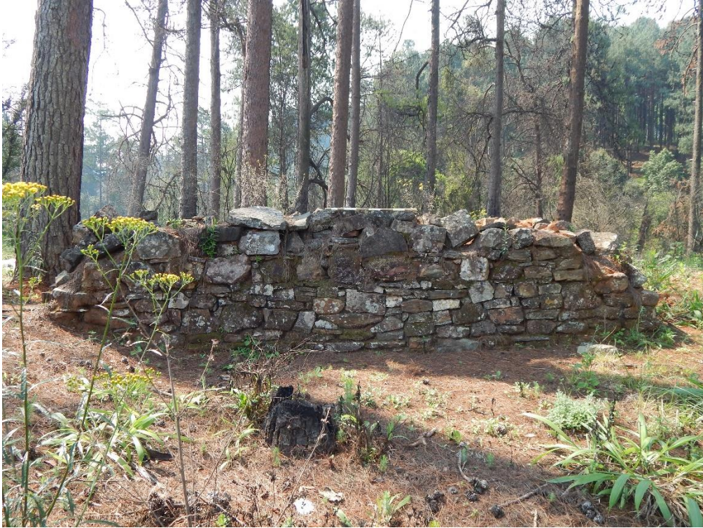
Fig. 5: The southern wall. Some damage occurred in this section, especially on the south-western and south-eastern corners.
