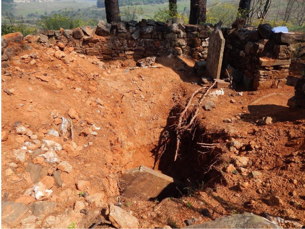
Fig. 13: Most of the excavated soil was piled up against the eastern wall.
