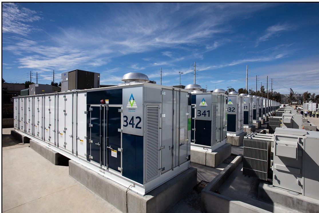
Figure 4: Close up view of a BESS (Photo: Greenbiz.com)
