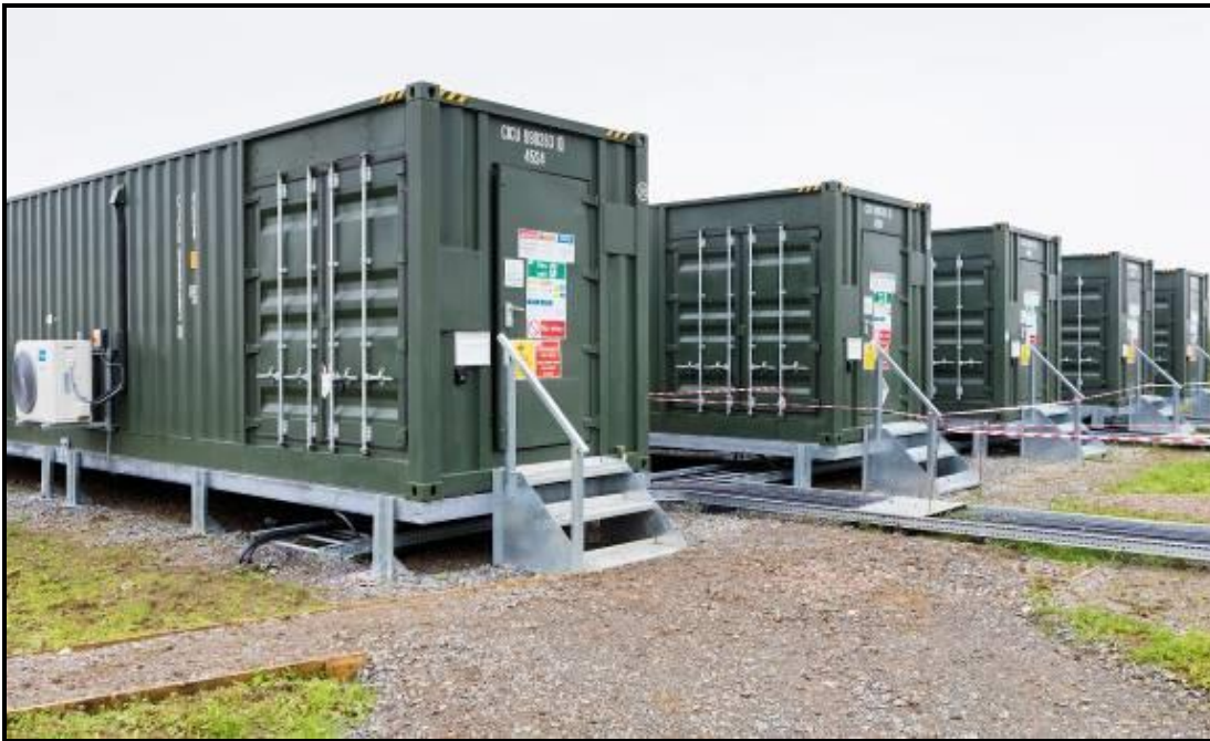
Photograph 1.2: Example of BESS located in storage containers
