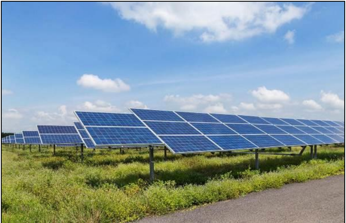
Photograph 1.1: Typical PV SEF facility
