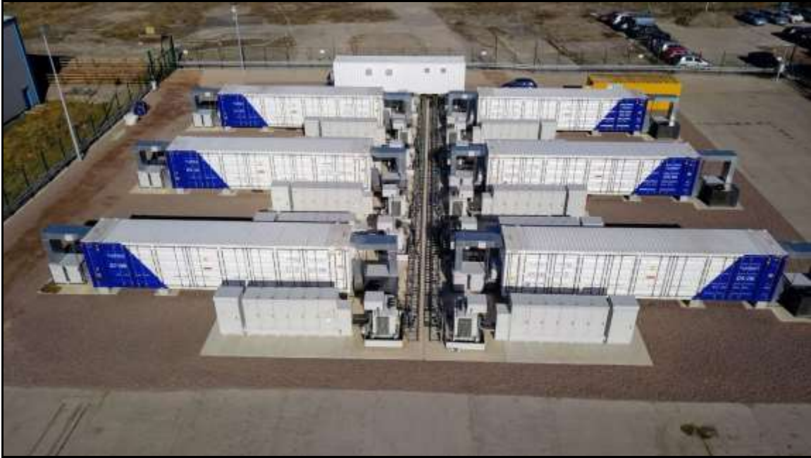
Photograph 1.2: Example of BESS located in storage containers
