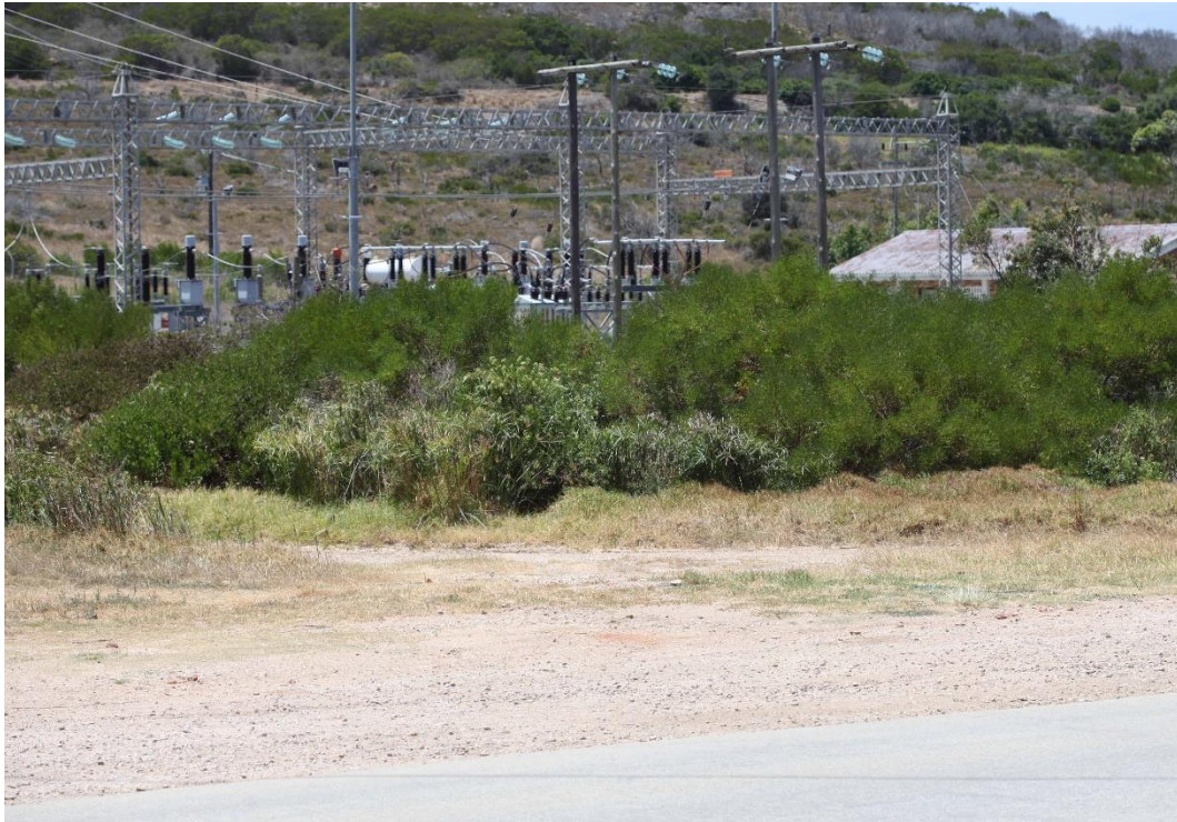
Photo 11 Road, watercourse (non-perennial river), riparian vegetation and substation north of the site. Photo: R.F. Terblanche.
