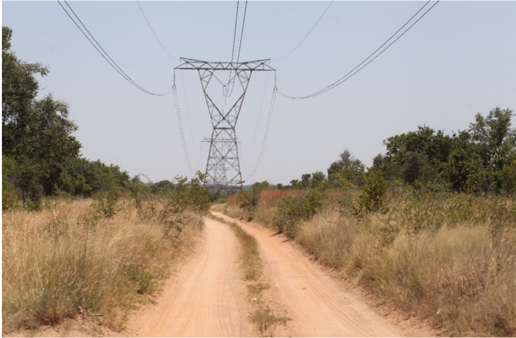
Photo 1 View, towards the south, along powerline at the eastern part of the site. Photo: R.F. Terblanche.
