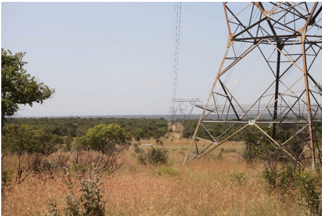
Photo 2 View, towards the north, along the powerline at the eastern part of the site. Photo: R.F. Terblanche
