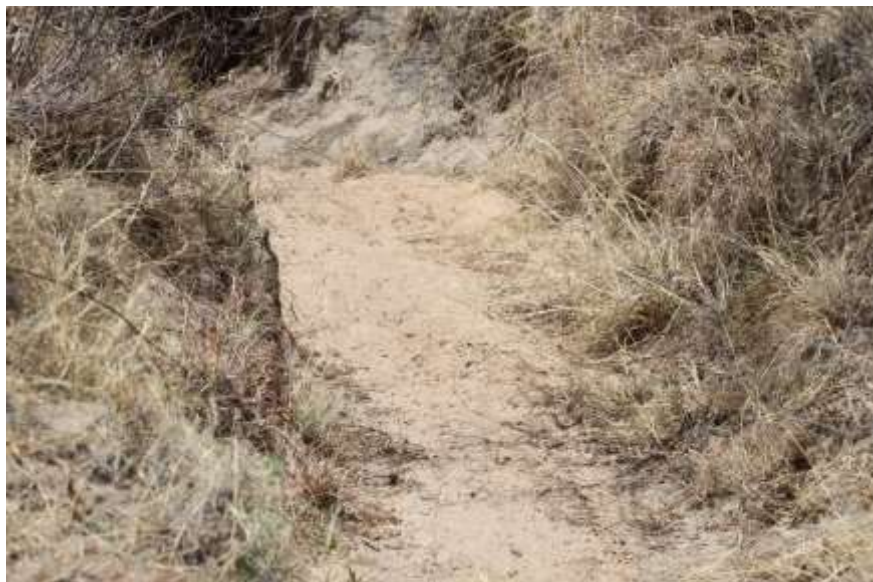
Narrow active channel at northern parts of the site. Photo: Reinier F. Terblanche.
