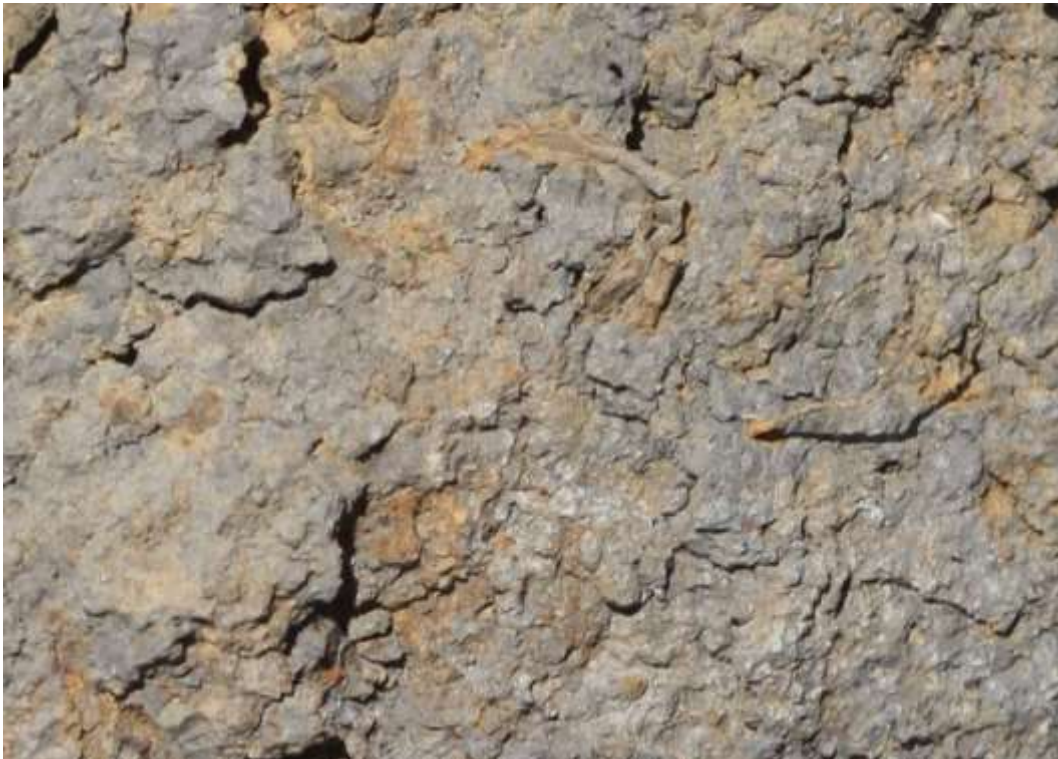
Photo 4 Soil that is seasonally inundated, at the site. Photo: R.F. Terblanche
