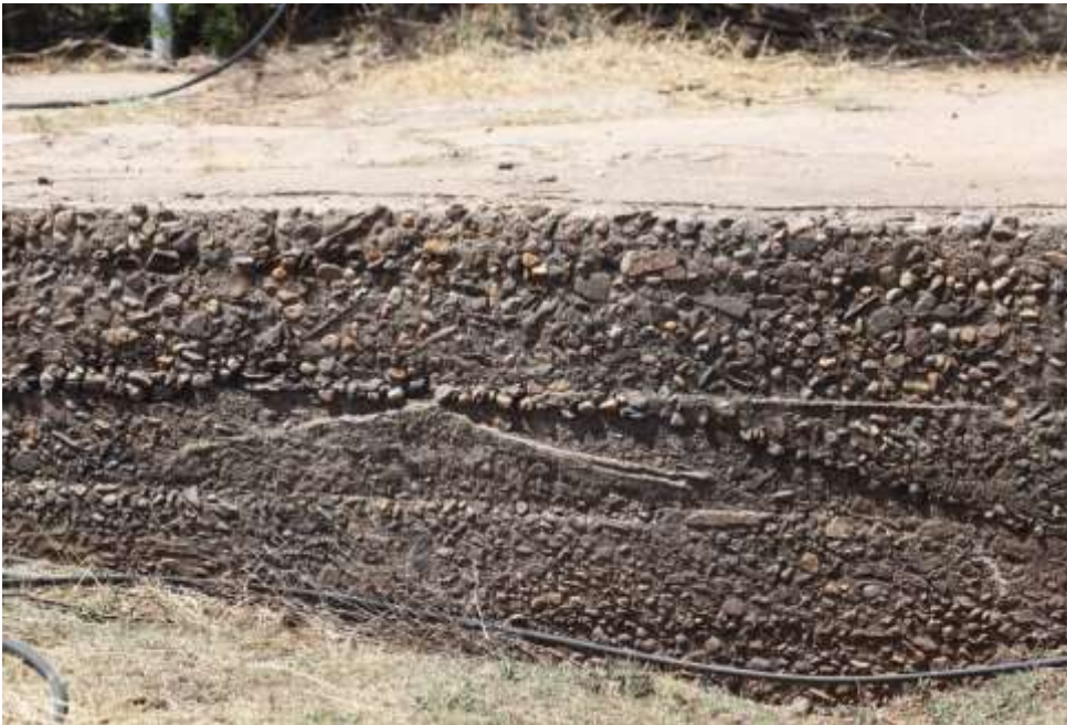
Photo 2 Low concrete wall where road crosses at the northeastern parts of the site, resulting in impoundment of water near an inlet of the Wentzel Dam.
