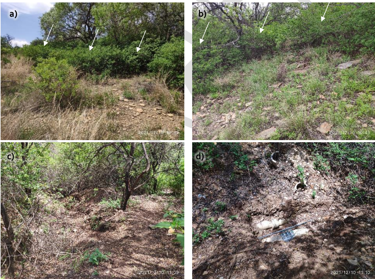
Photograph 4: a & b) Almost impenetrable Lantana camara infestation around the edges of a dense tree canopy c) eroded or dug up pipeline route within the dense tree canopy, just beyond the Lantana edges and d) exposed pipeline route
