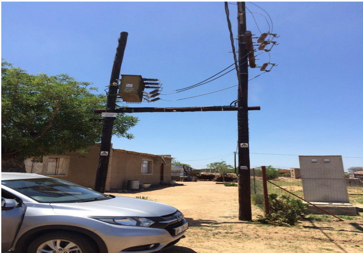
Picture: Shows the existing transformer on site
