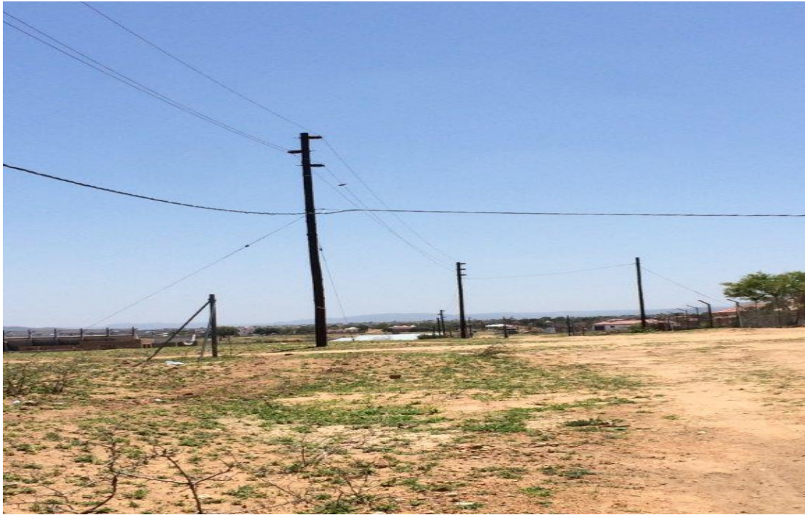
Picture 1: Shows the existing MV lines on site
