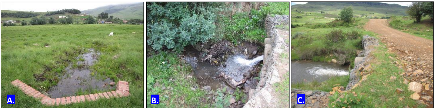
(a): Brick culvert at watercourse crossing 10 (b): Pipe directing water underneath main road at watercourse crossing 8 (c): The existing culvert across the Mooi River (WC 11). The proposed pipes will be tied to these structures.
