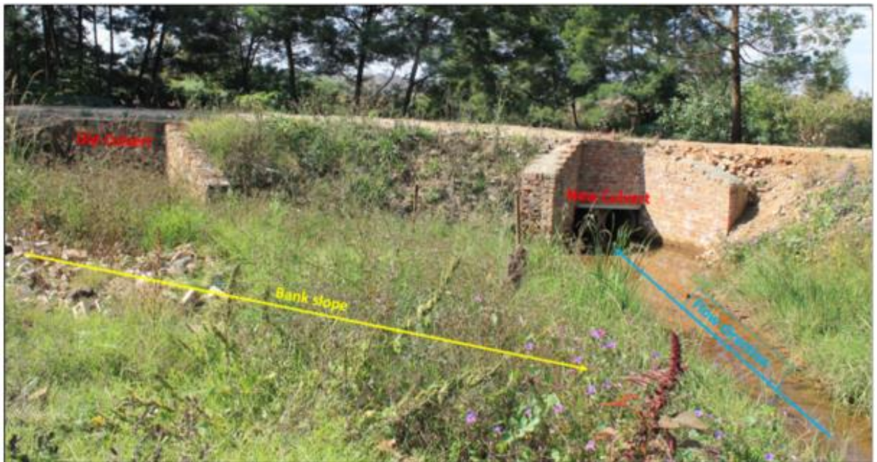
Figure 5-3: The position of the newly constructed culvert and the old culvert (TBC, 2022)
