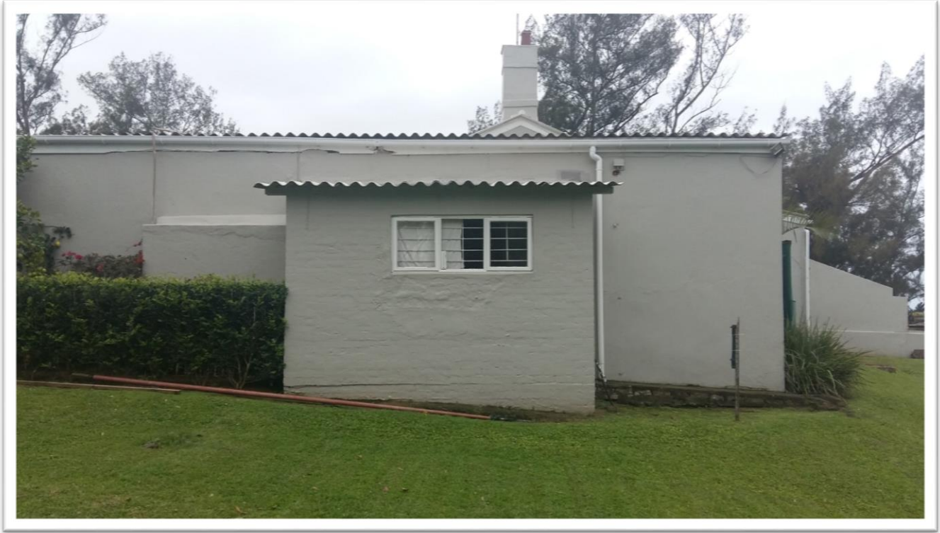
Garage with demolished chimney protruding on the left of the older outhouse structure.
