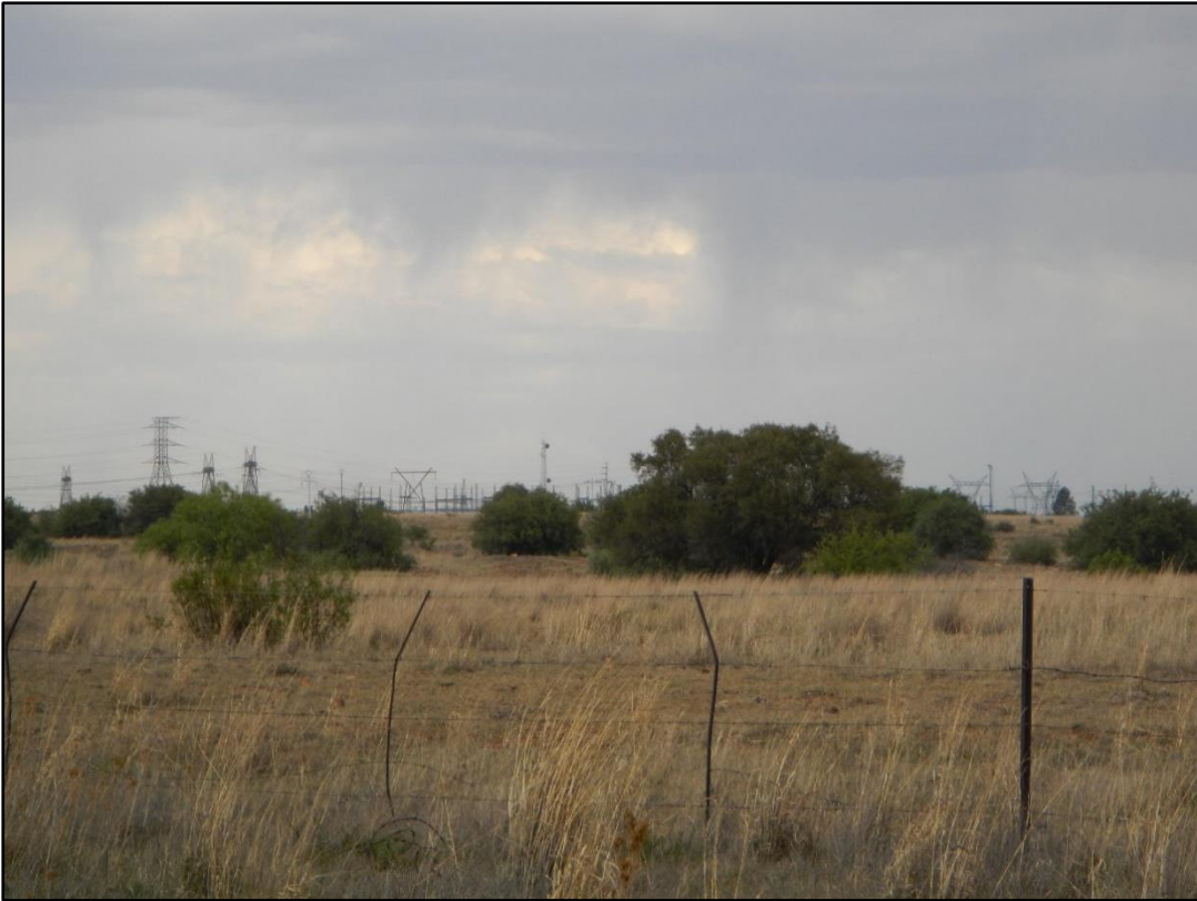
Figure 6: Tall steel structures that make up the Watershed MTS, as well as the tall steel towers of the existing 132kV power lines that run to the Watershed MTS, which can be seen from various parts of the surrounding area
