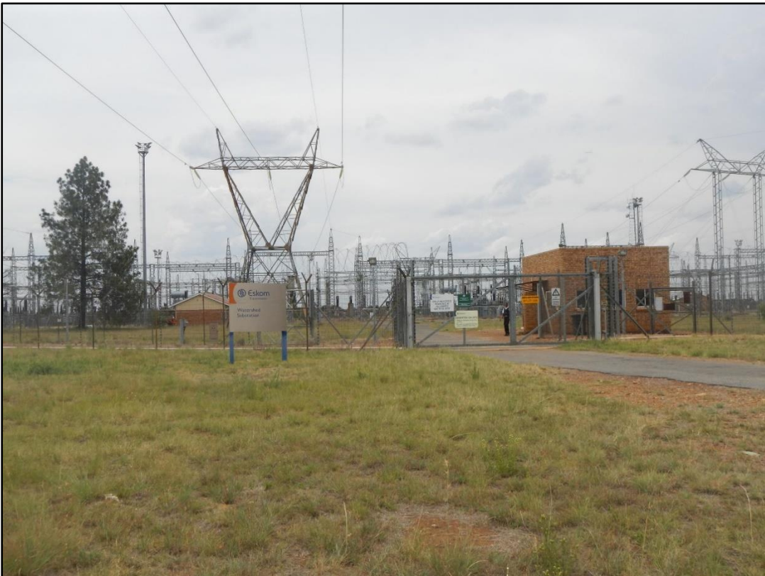
Figure 7: View of the Watershed Main Transmission Substation (MTS), which can be found within the corridor
