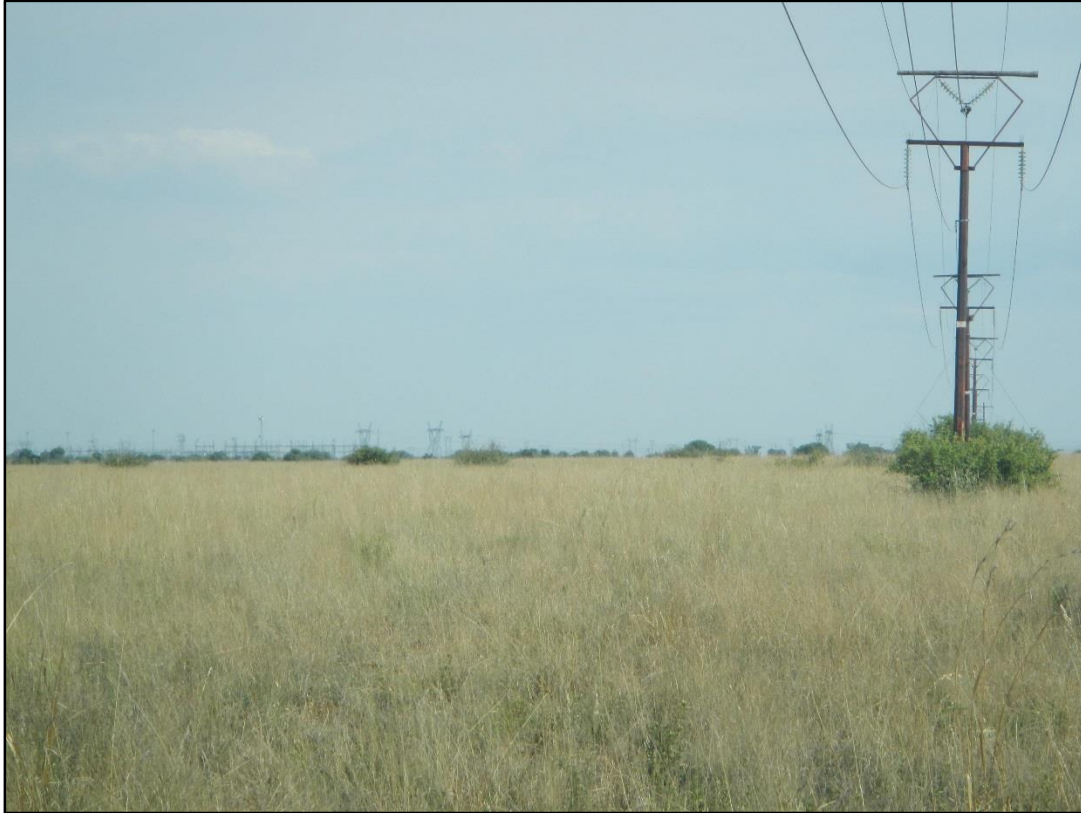
Figure 21: The tall steel structures of the Watershed MTS which can be seen from certain parts of the Lichtenburg Game Breeding Centre.
