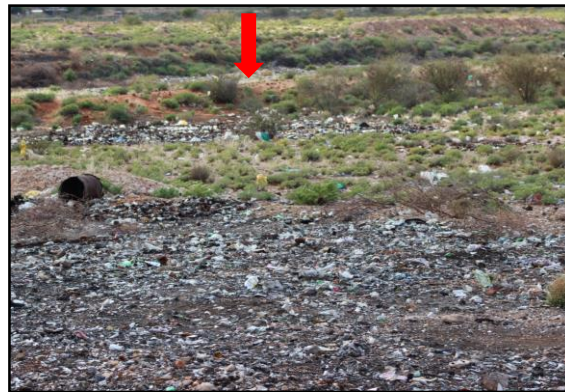
Figure 3: View north east towards the cell indicated by red arrow. Note waste strewn outside the cell (July 2015)
