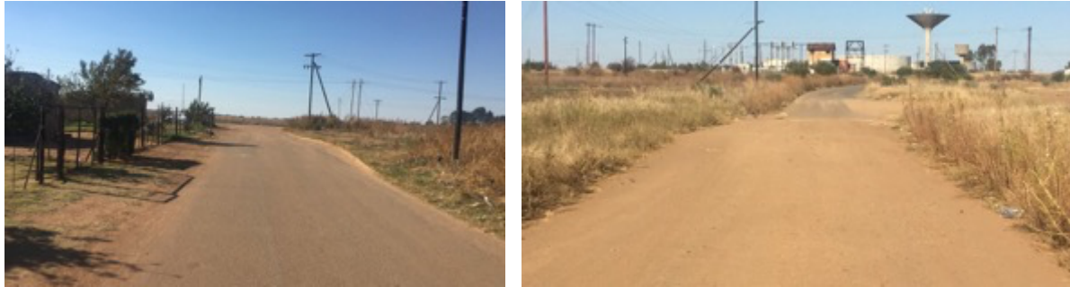
Figure 13 – Intersection C – Road Condition
