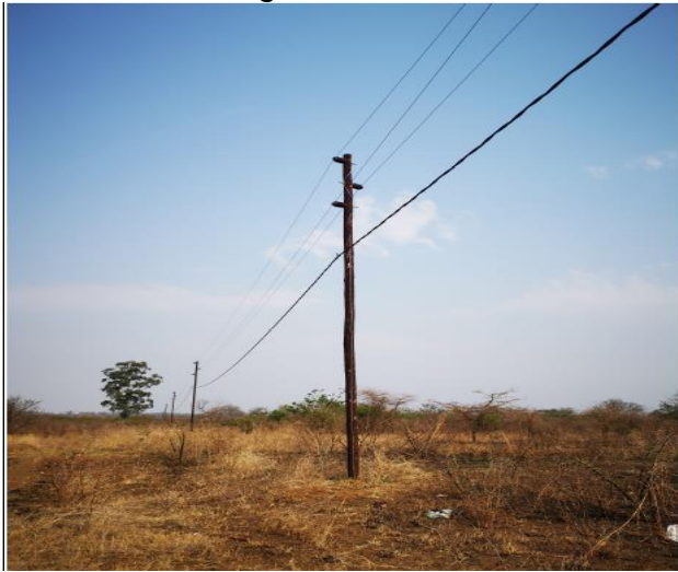
Existing MV Feeder line
